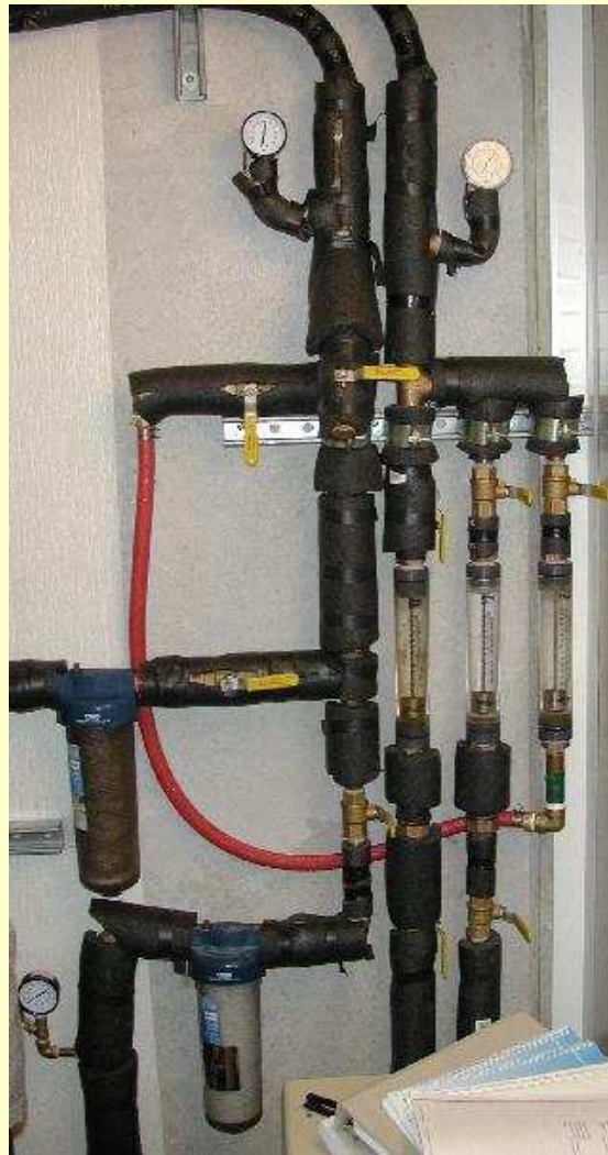
Inside Laser Room
